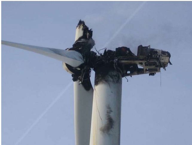
Fig. 2: Burnt down nacelle of a 1.5 MW wind turbine (Image source: Allianz)
