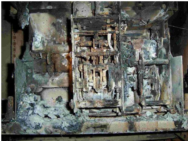
Fig. 3: Power switch of a 1 MW wind turbine – destroyed by fire (Image source: Allianz)
